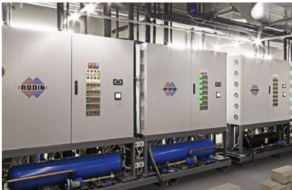
Figure 4 C-Town Rack System
