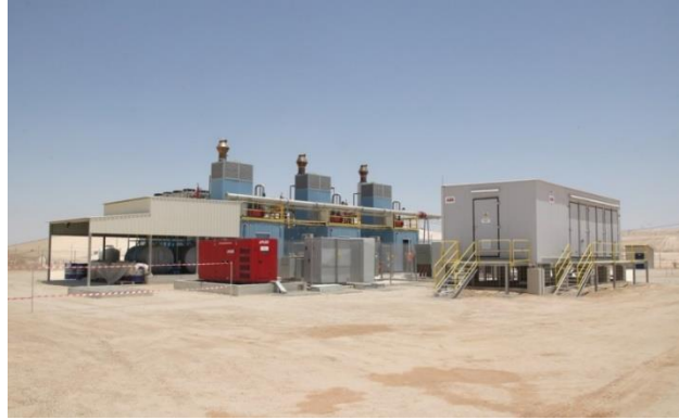
Figure 17: CHP unit in Al-Gabawi Landfill.
